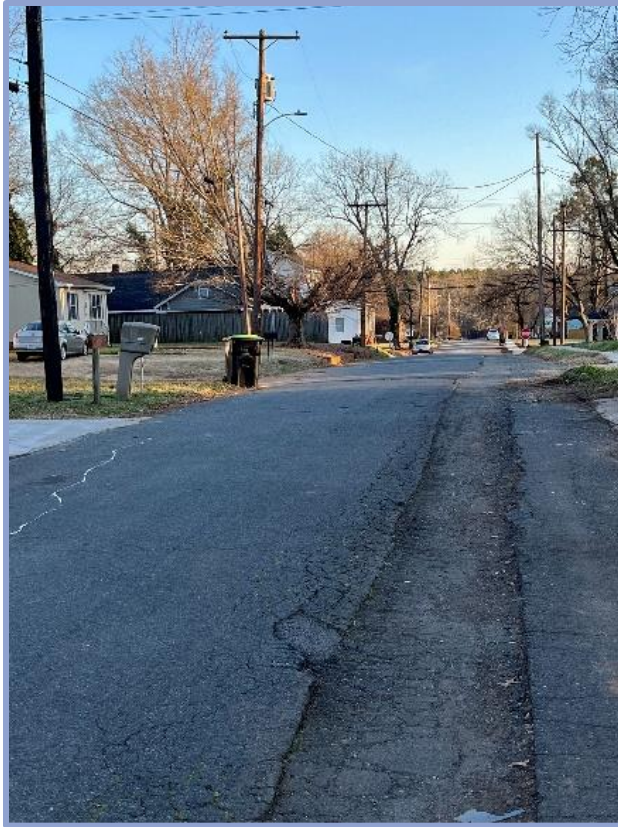
Figure 12: Damaged Infrastructure on Long Street Highlights Vulnerabilities
